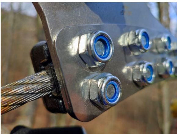
Non-compliant screw assembly
